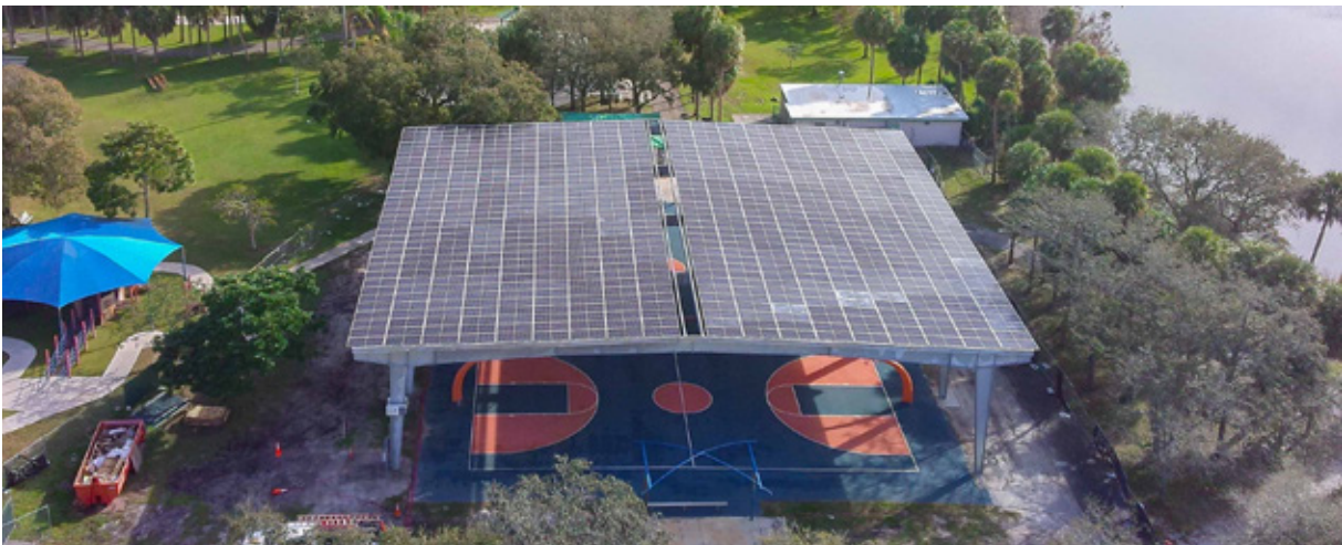
Two large-scale solar canopies over the basketball courts at Reverend Samuel Delevoe Memorial Park in Fort Lauderdale.
